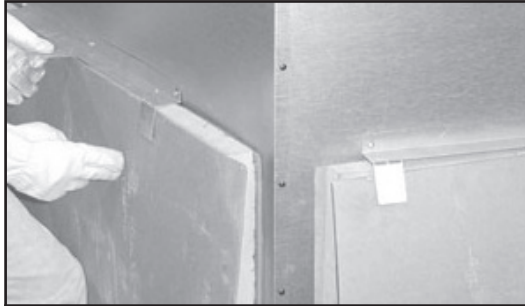
Figure 3.6 Unpack Back Refractory
