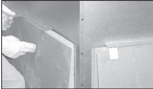
Figure 3.6 Unpack Back Refractory
