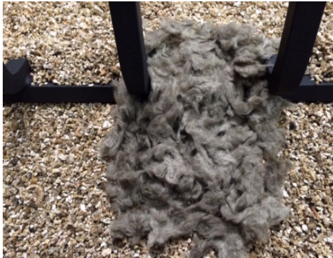
Figure 5c- Carry over tube covered by rock wool
