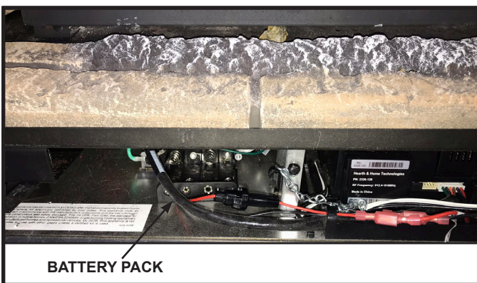
Figure 3.8 Battery Pack Installed
