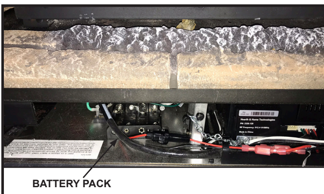
Figure 3.8 Battery Pack Installed
