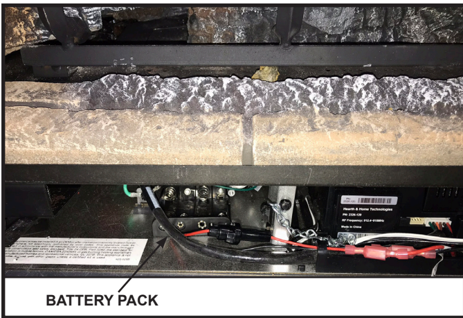
Figure 6.3 Battery Pack Installed
