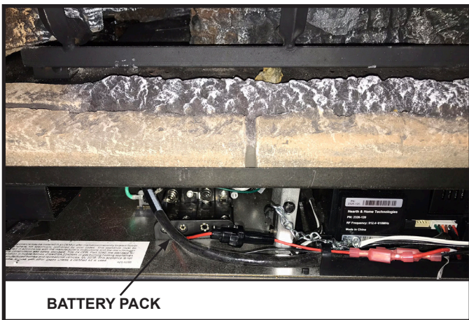
Figure 6.3 Battery Pack Installed
