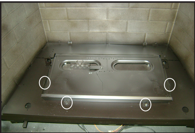
Figure 4.10 Remove Burner Skirt
