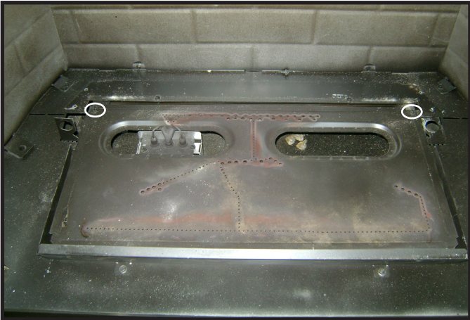
Figure 4.9 Remove Screws from Burner Assembly Rear Corners
