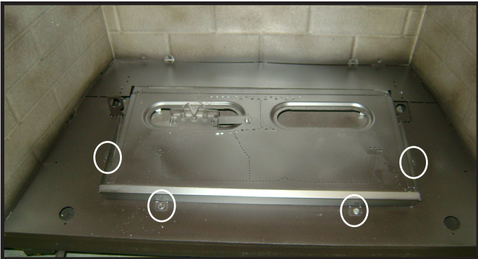
Figure 4.10 Remove Burner Skirt
