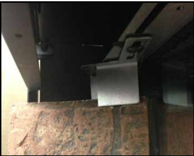
Figure 11.28 Side Refractory Brackets
