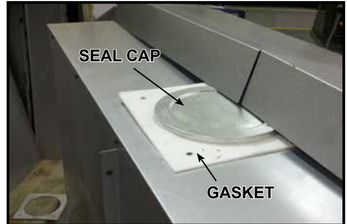
Figure 6.2 Seal Cap and Gasket Location
