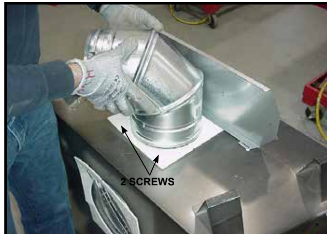
Figure 6.11 To attach the first section of vent pipe, make sure to use the fiberglass gasket to seal between the first vent component and the outer fireplace wrap. Use 2 self tapping screws to secure the gasket to the outer wrap.
